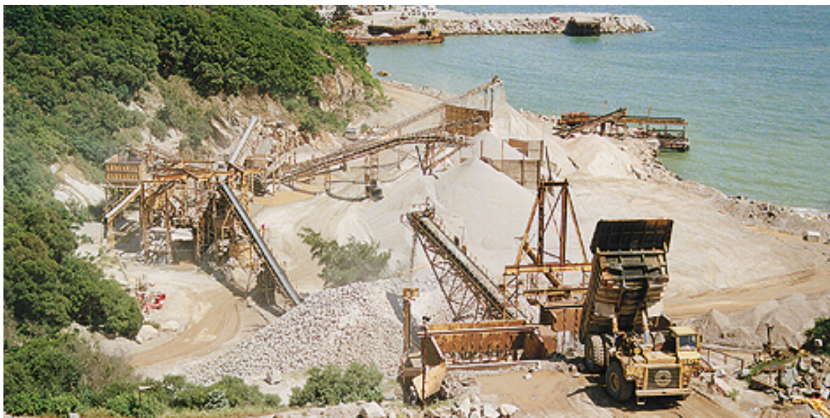
Crushing Plant at Niu Tou Quarry, Zhuhai, PRC
